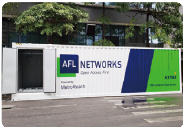
Container data center in Nigeria
