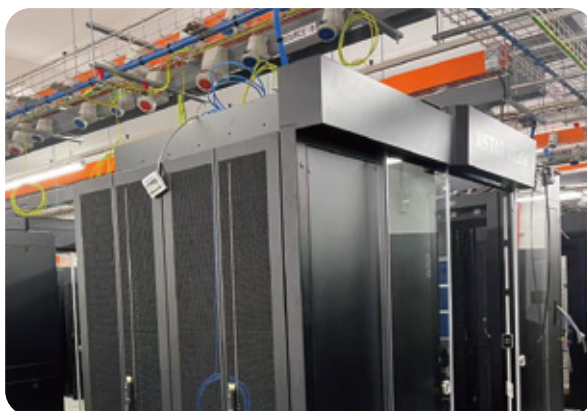
An enterprise datacenter in Singapore
