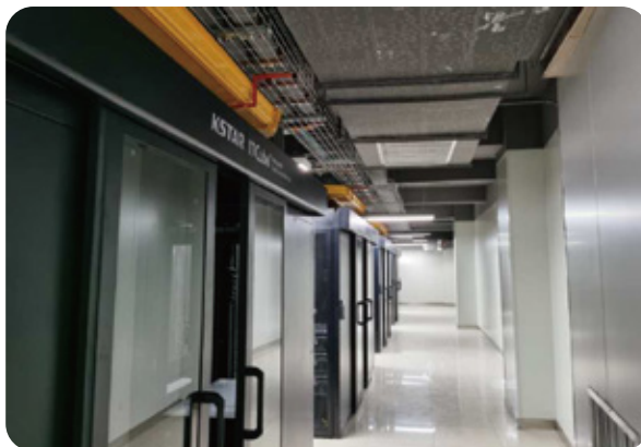
A data center in Jiangyou, Sichuan Province
