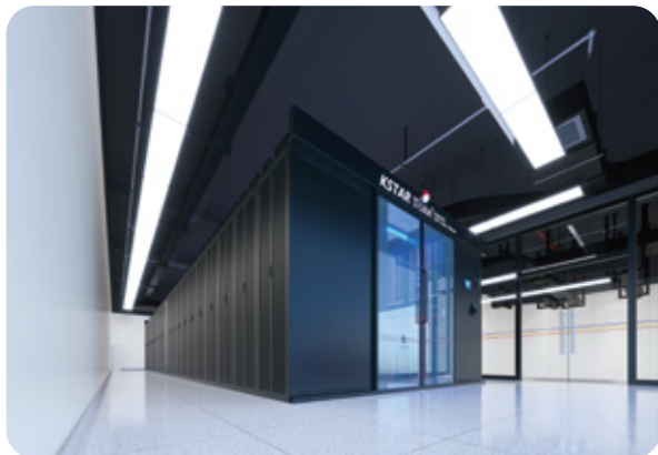
An enterprise data center in Shaanxi Province
