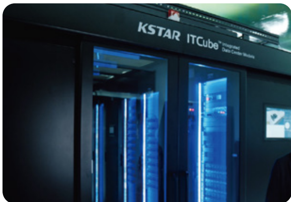
Malaysian Prime Minister's Department Data Center
